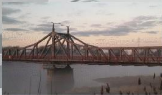
The steel bridge over the Oder River in Krosno Odrzańskie. The bridge was fabricated at Georg Beuchelt's works in Grünberg (presently Zielona Góra).
