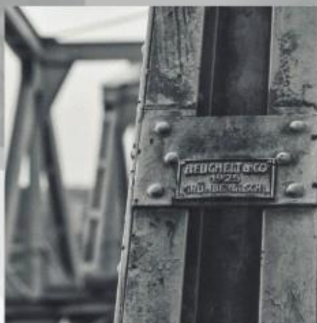
The steel bridge over the Oder River in Kędzierzyn-Koźle (Silesia). The bridge was fabricated at Georg Beuchelt's works in Grünberg (presently Zielona Góra).
